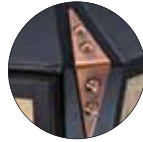
Washed Copper Detail Shown
